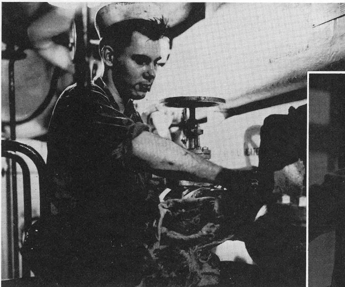
Cutting in the fuel oil heater
